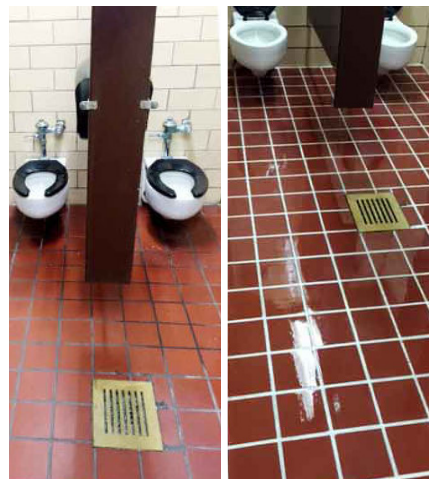
Quarry Tile & Grout Coated With X-PROTECT PERFORMANCE TOPCOAT - High Gloss (John Deere Facility/ Before & After Comparison)
